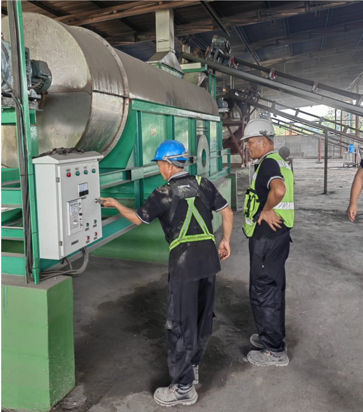
Figure 2: The PYX team inspecting the installation of a new dryer machine at our mineral separation plant at Mandiri.
